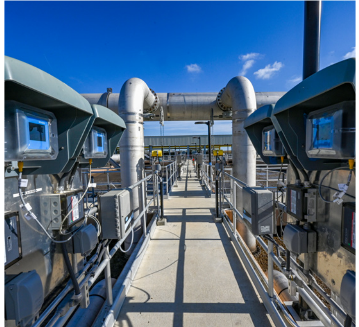
Public Utilities brings the Bee Ridge Advanced Water Treatment Facility online.
