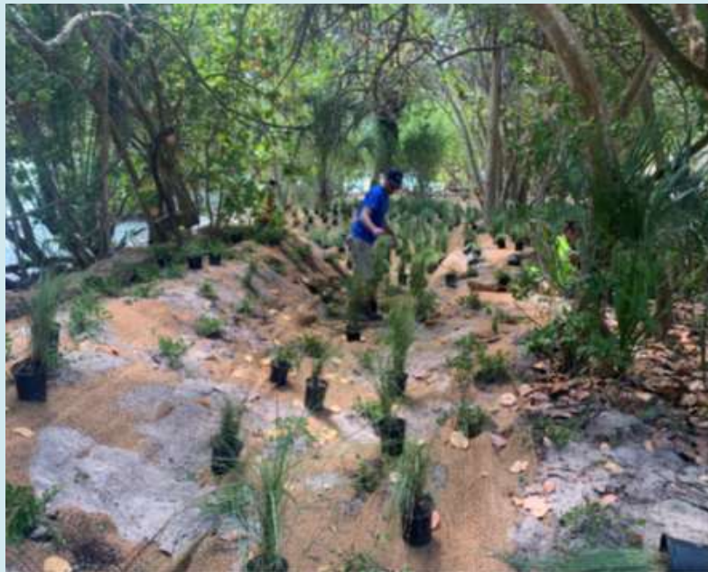
Vegetated, terraced spillway with erosion control mat.
