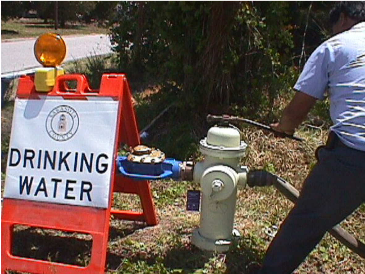
Extension of Water Lines to Areas Served by Potable Water Wells is a Priority in Nokomis
